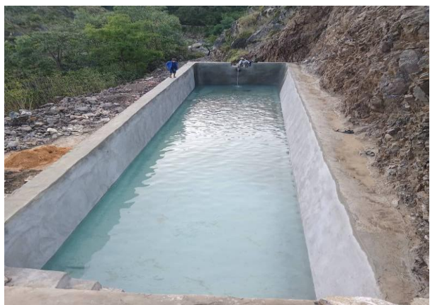
Water Harvesting Tank in Al-Taweelah – Al-Mahweet.
